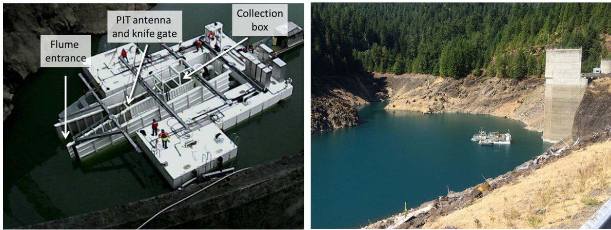
Figure 31. Photographs showing portable floating fish collector in Cougar Reservoir during construction with pertinent features (left) and position of the portable floating fish collector relative to the water temperature control tower in the cul-de-sac of Cougar Dam and Reservoir (right), South Fork McKenzie River, Oregon, July 2015. Left photograph by Collin D. Smith, U.S. Geological Survey, March 26, 2014; right photograph by Jamie M. Sprando, U.S. Geological Survey, July 28, 2015.
